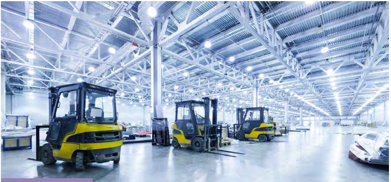
LED lighting in a warehouse
