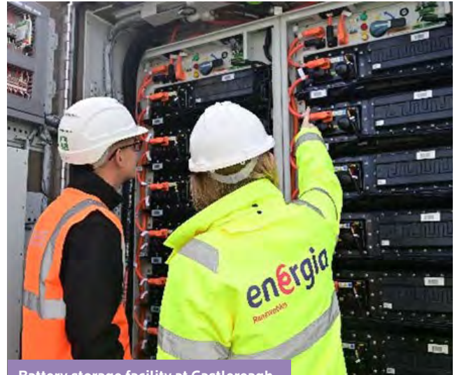
Battery storage facility at Castlereaigh
